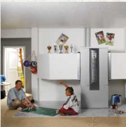
Air/Water heatpump indoor installation 26 kW
