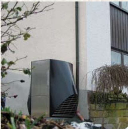
Air/Water heatpump outdoor installation 33 kW
